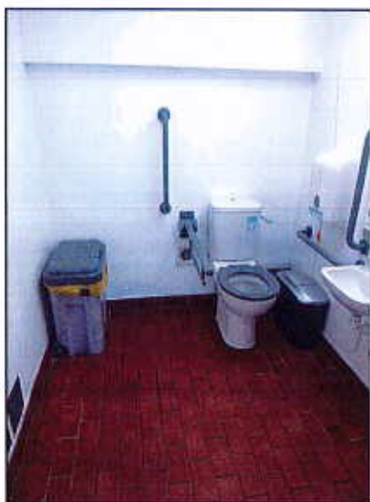
Image 18: Accessible toilet showing a sanitary bin in the wheelchair recess and inaccessible alarm cord
