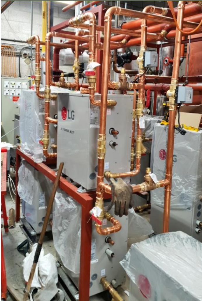
Hydro boxes – transferring heat from outside
